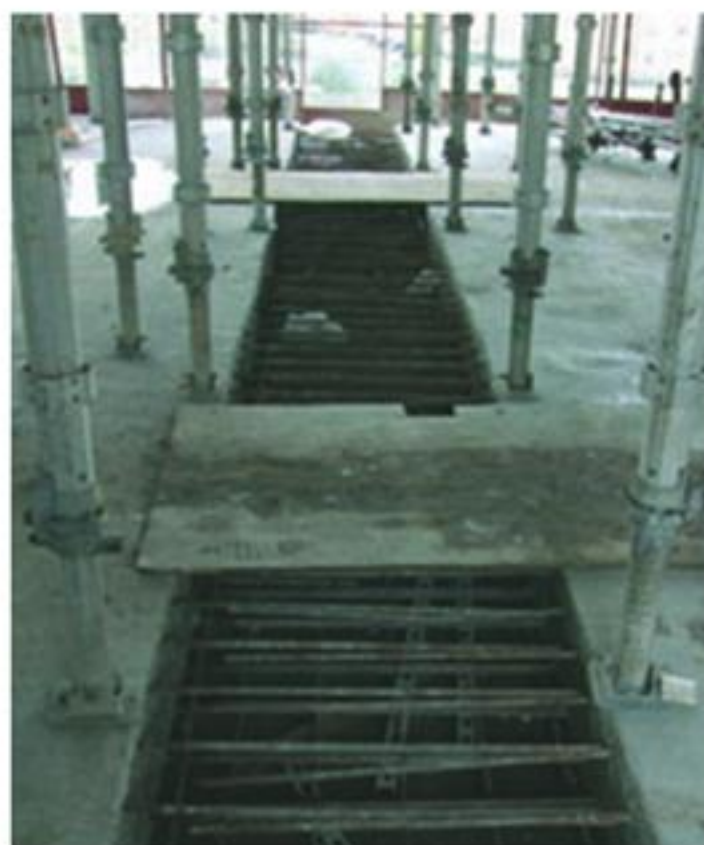
Pour Strips restrict site access, cause a trip hazard and delay progress on site
