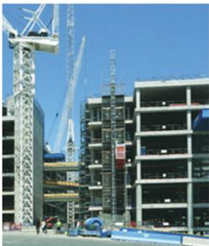
5,000 Lockable dowels were installed on the Royal Children's Hospital in Melbourne, Australia
