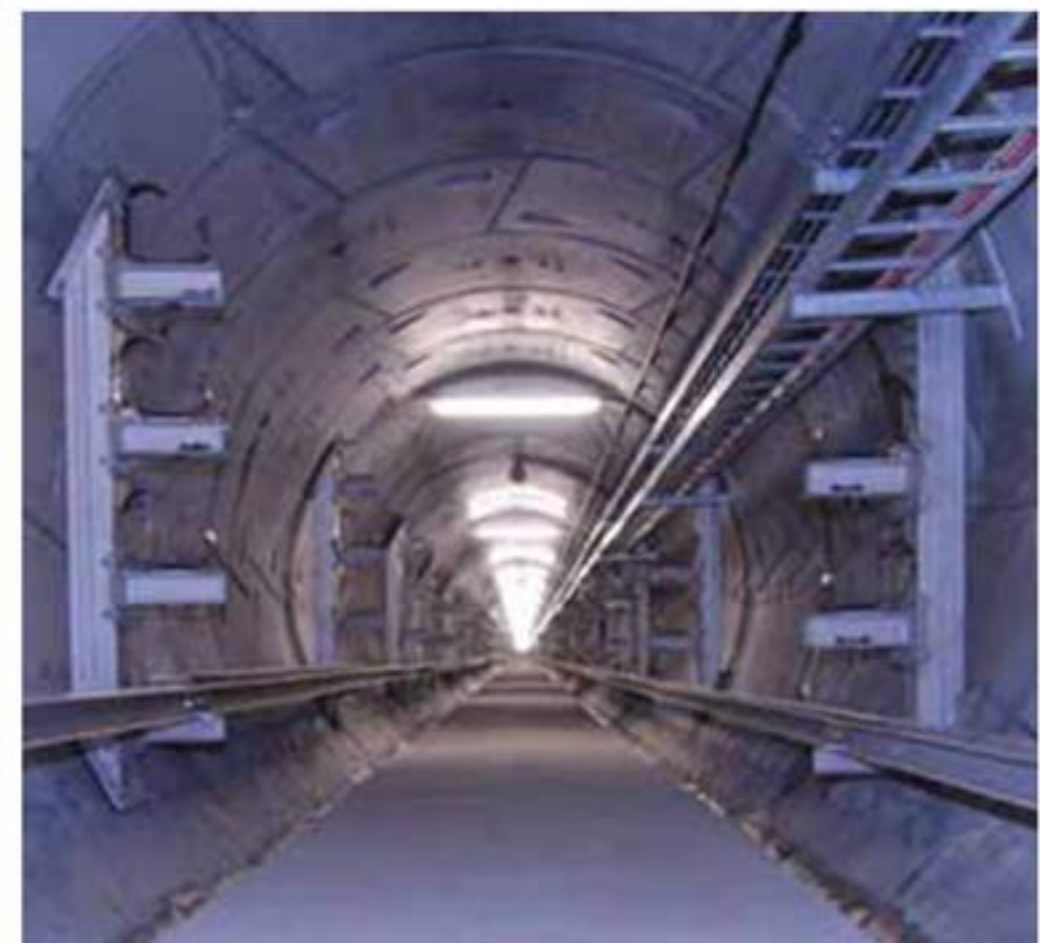
Project: City West Cable Tunnel, Australia (Client: Energy Australia, Contractor: Thiess, Engineer: Maunsell/AEcom)
