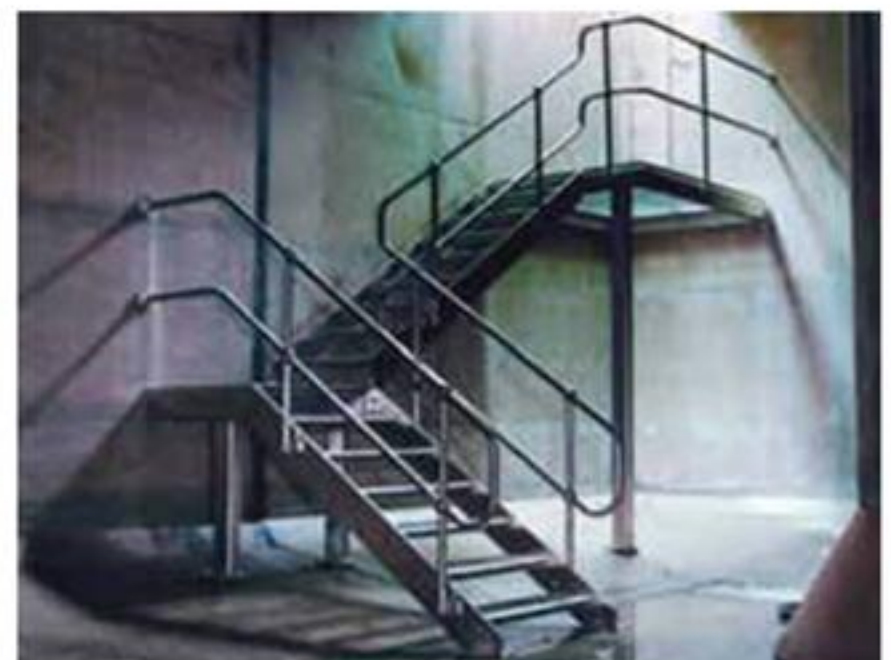
Access Walkways and Ladders
