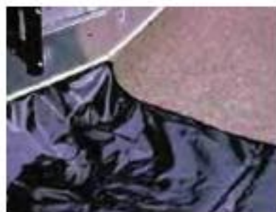
The moisture mat being installed over the root barrier and secured at the roof perimeter.
