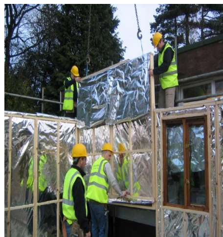
Eco-Brite installed in prefabricated wall panels
