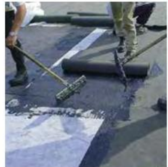
4. Laying the Hydrogard protection layer over second coat of Hydrotech Monolithic Membrane 6125
